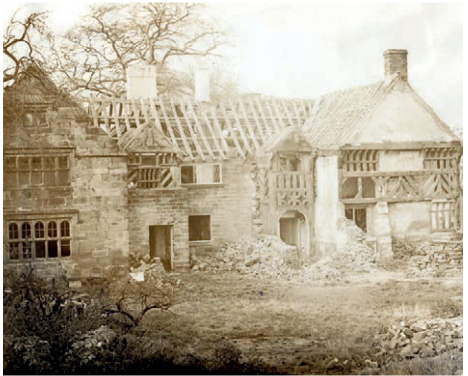
Gawber Hall, Barnsley being demolished in 1935. Courtesy of Barnsley Metropolitan Borough Council
